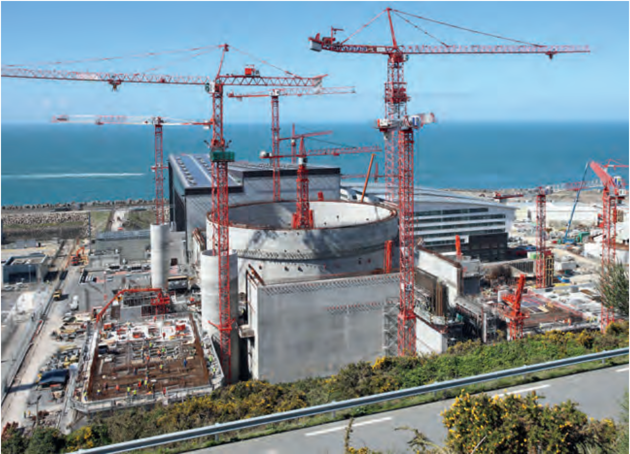
••• IRSN was involved in monitoring progress in construction work on the Flamanville 3 reactor in Normandy.
