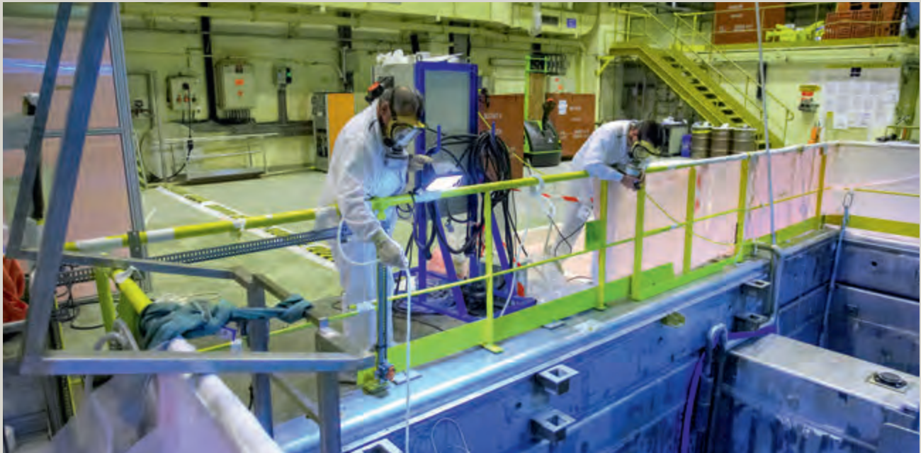
•• In 2011, IRSN examined the safety review documentation for the CEA's MAR 400 decladding unit in Marcoule in southern France.
