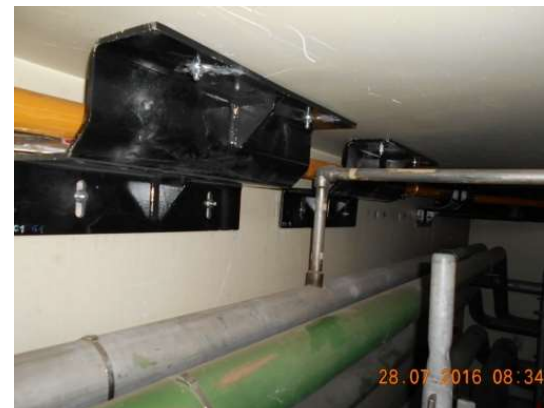
AGRESSION EXPLOSION INTERNE Protections tuyauteries
