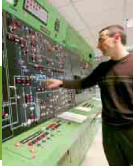
Control room of the DIVA experimental installation.
