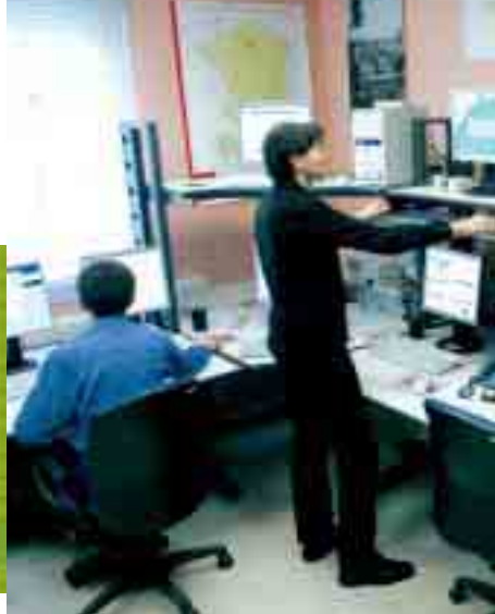
Real-time radiological monitoring of French territory in the warning systems remote monitoring room in Le Vésinet (Yvelines).
