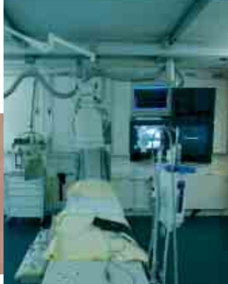
Cardiological radiology installation at Cochin Hospital.
