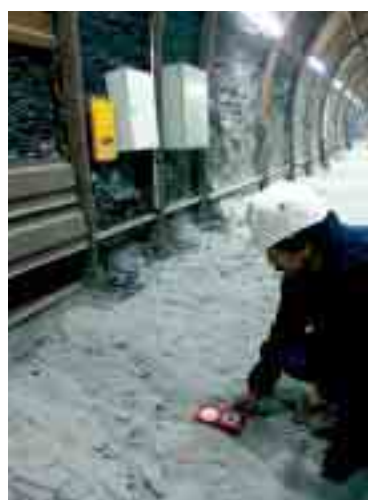
Measuring the direction of cracks in a tunnel gallery at Tournemire (Aveyron).
