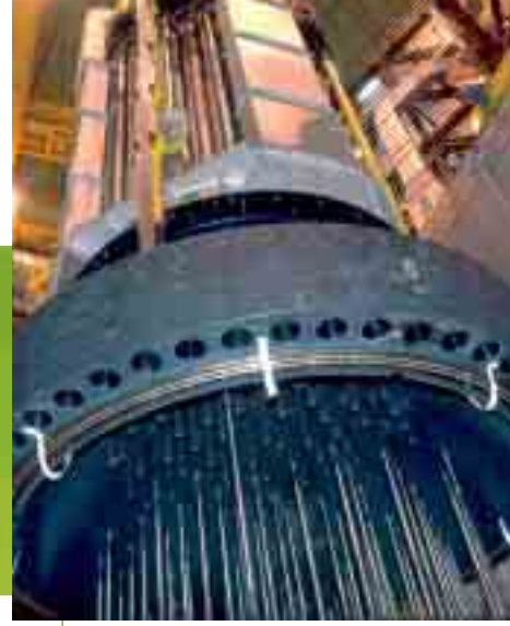
Reactor vessel head at the Civaux power plant (Vienne).
