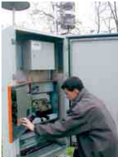
Inside a SARA monitor (automated aerosol radioactivity monitoring device).
