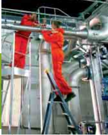
Ventilation system at the DIVA experimental installation at Cadarache (Bouches-du-Rhône).
