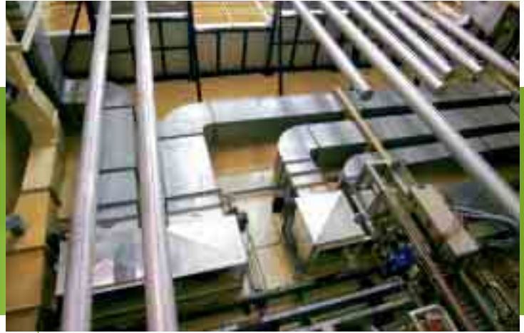
PHEBUS reactor: dry storage area for test devices.
