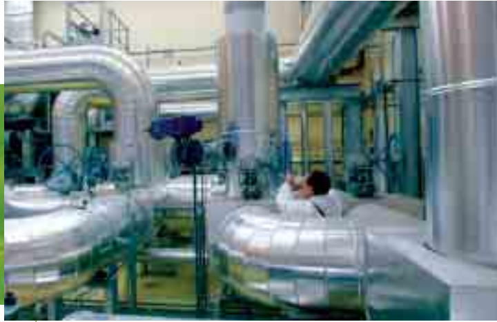
Full-scale blowing device to test the strength of VHE filters and fire dampers under pressure (STARMANIA).
