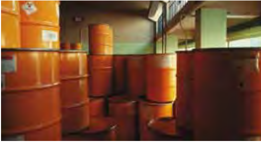
Interim storage of waste in a hall of the Brennilis power plant (EDF).
