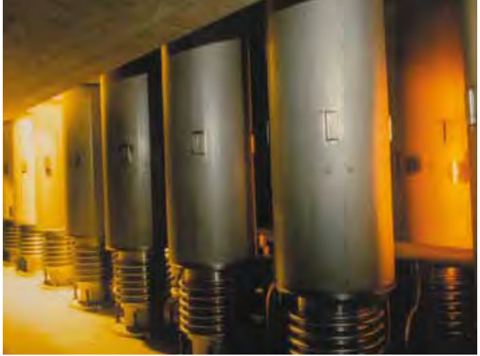
Interim vitrified waste storage. View in the lower part of the shafts (La Hague).
