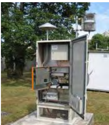
Figure 27 : Photo de la station SARA
