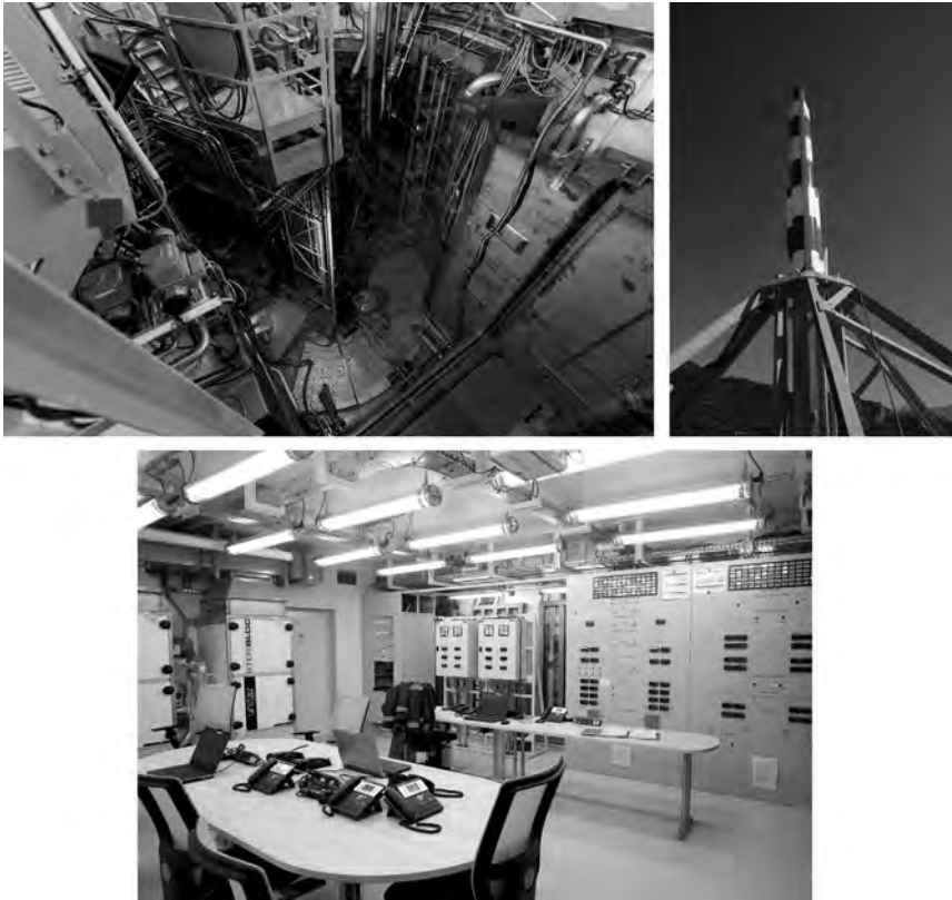
Figure 10.9. Three measures selected for the RHF at Grenoble after the Fukushima Daiichi accident, all designed and sized for extreme earthquakes and flooding: on the top left, the pool inlet elbow of the groundwater supply system. © IRSN; on the top right, the seismic depressurization system stack positioned on the dome of the metal containment. © ILL; at the bottom, the PCS 3 emergency control room. © Jean-Marie Huron/Signatures/IRSN.
