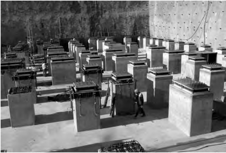
Figure 7.11. View of aseismic bearing pads during construction of the Jules Horowitz reactor (2009), from “ Le Blog des Énergies ”. © DR.
