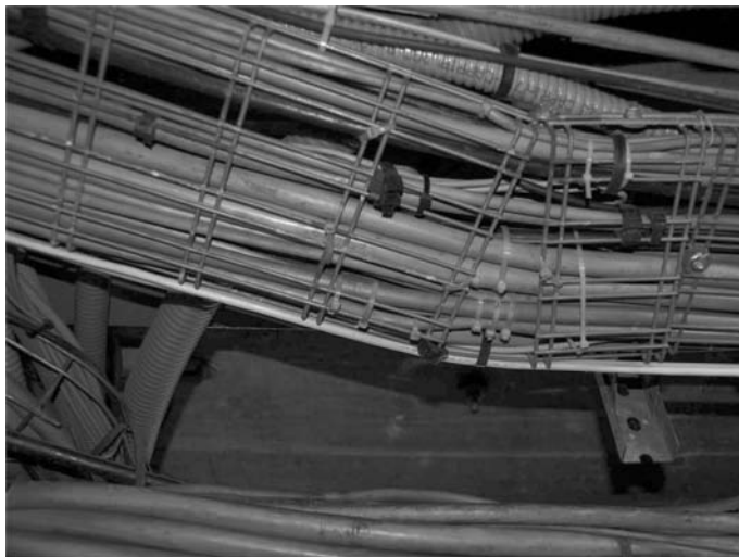
Figure 7.1 Example of a cableway configuration in an installation. @ Georges Goué/IRSN.
