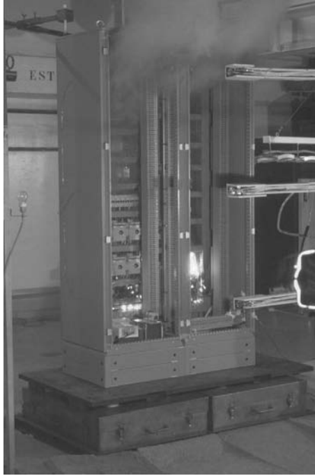
Figure 7.4 Fire in a type of electrical cabinet used in fuel cycle installations, tested at the SATURNE facility as part of the PICSEL program. © Florent-Frédéric Vigroux/IRSN.
