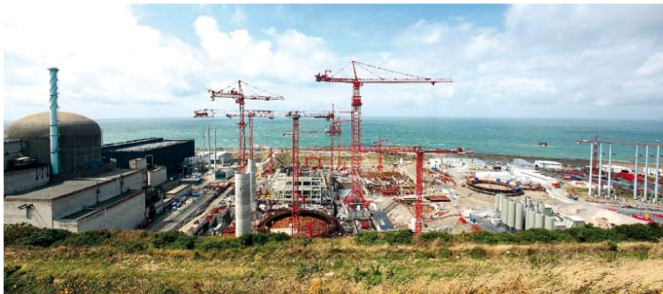
During inspections conducted by the ASN, IRSN experts detected cases of non-compliance on the EPR worksite.
